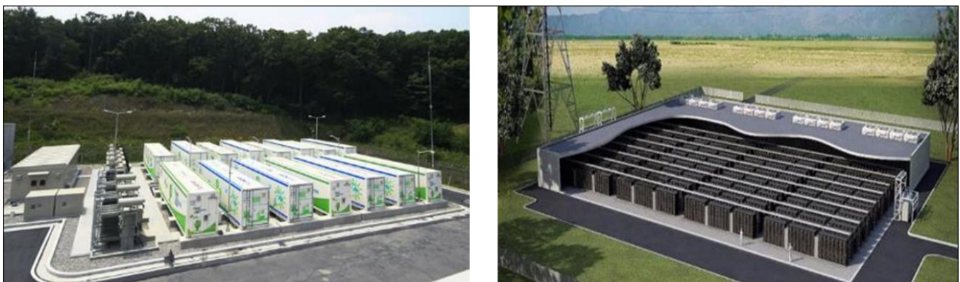
Figure 9 Battery Energy Storage System (BESS)
