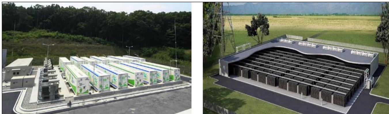
Figure 9 Battery Energy Storage System (BESS)
