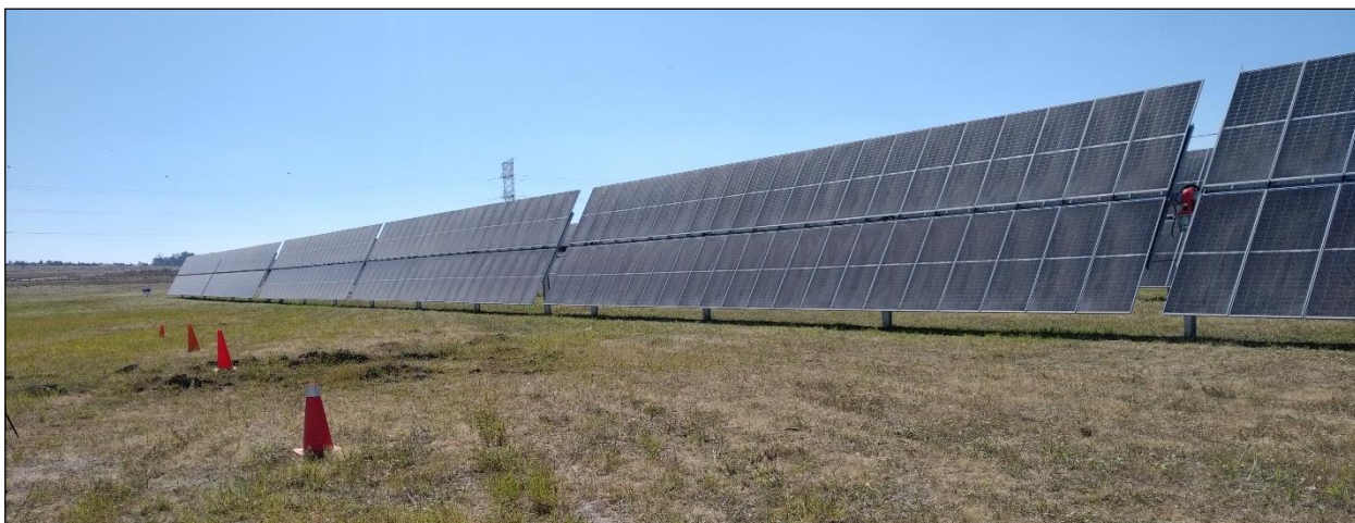
Figure 8 Front views of the PV arrays mounted on horizontal 1-axis tracker
