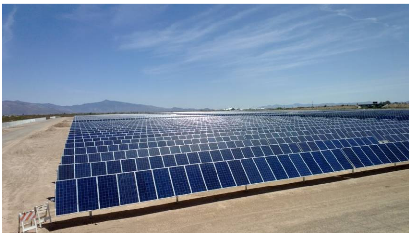
Figure 4: Illustration of tracking PV technology panels
