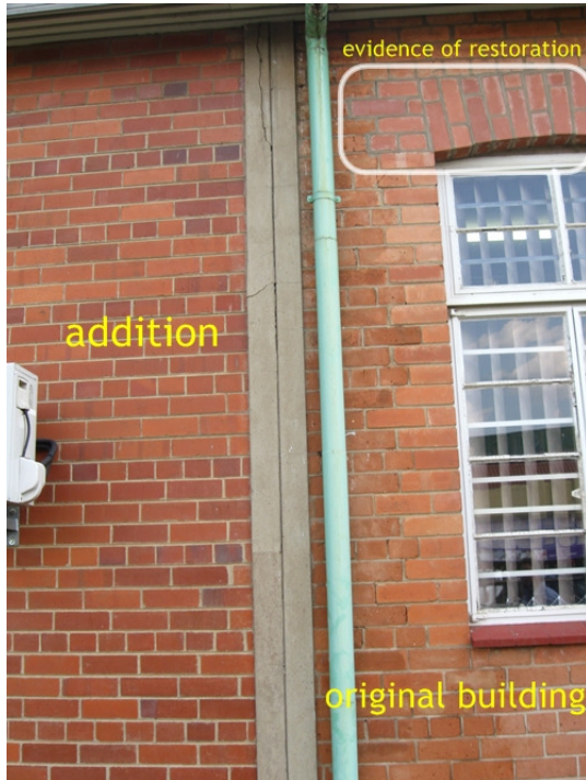
Image 3: Illustrates the existing part of the building as well as the addition. There is a visible difference in the different bricks used and new brickwork is also visible over the existing windows.
