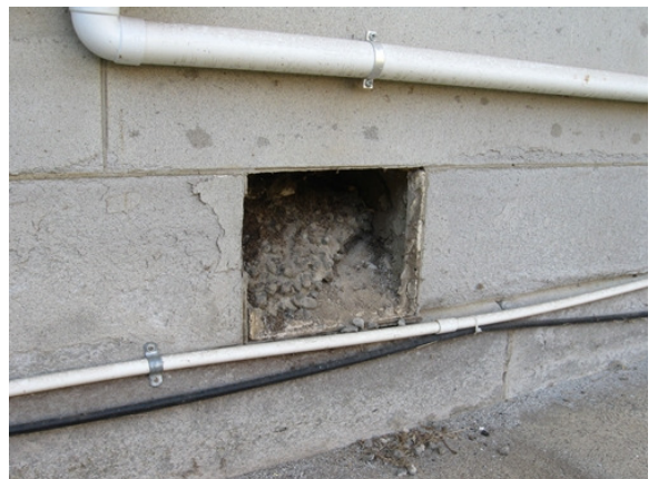
Image 34: Damaged floor vent
