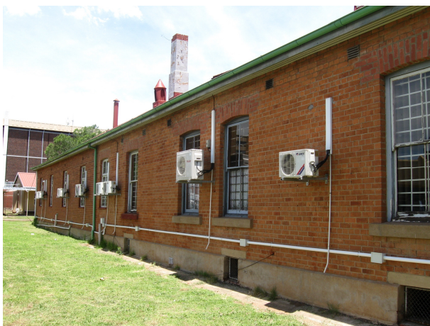
Image 25: Illustrating the harsh effect of the air-conditioning units on the elevation.
