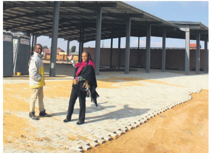
Construction work on a municipal vehicle parking depot has been delayed yet again. Seen at the depot are the project's community liaison officer Sello Malaka and Ward 78 cllr Zanele Nyakale.
