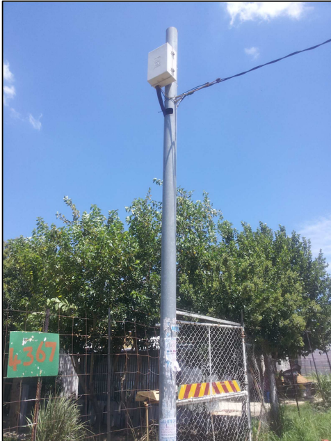
Figure 3: Existing lighting control box
