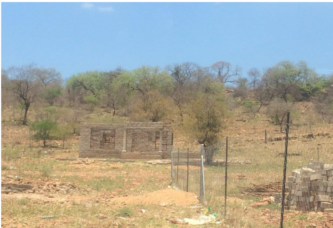
Picture 6 : Shows other unfinished houses on site
