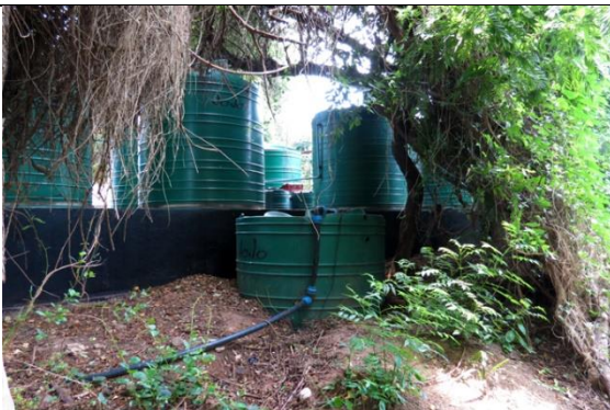
Water treatment facility
