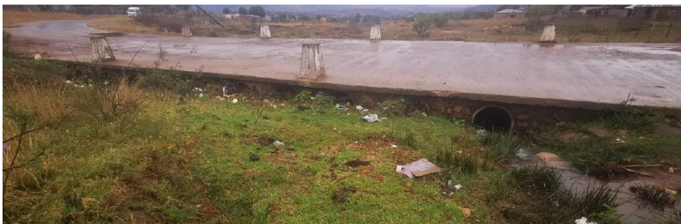
Figure 6 Stream 2, culvert 2, barrels 10No. 600mm pipe culvert, blocked
