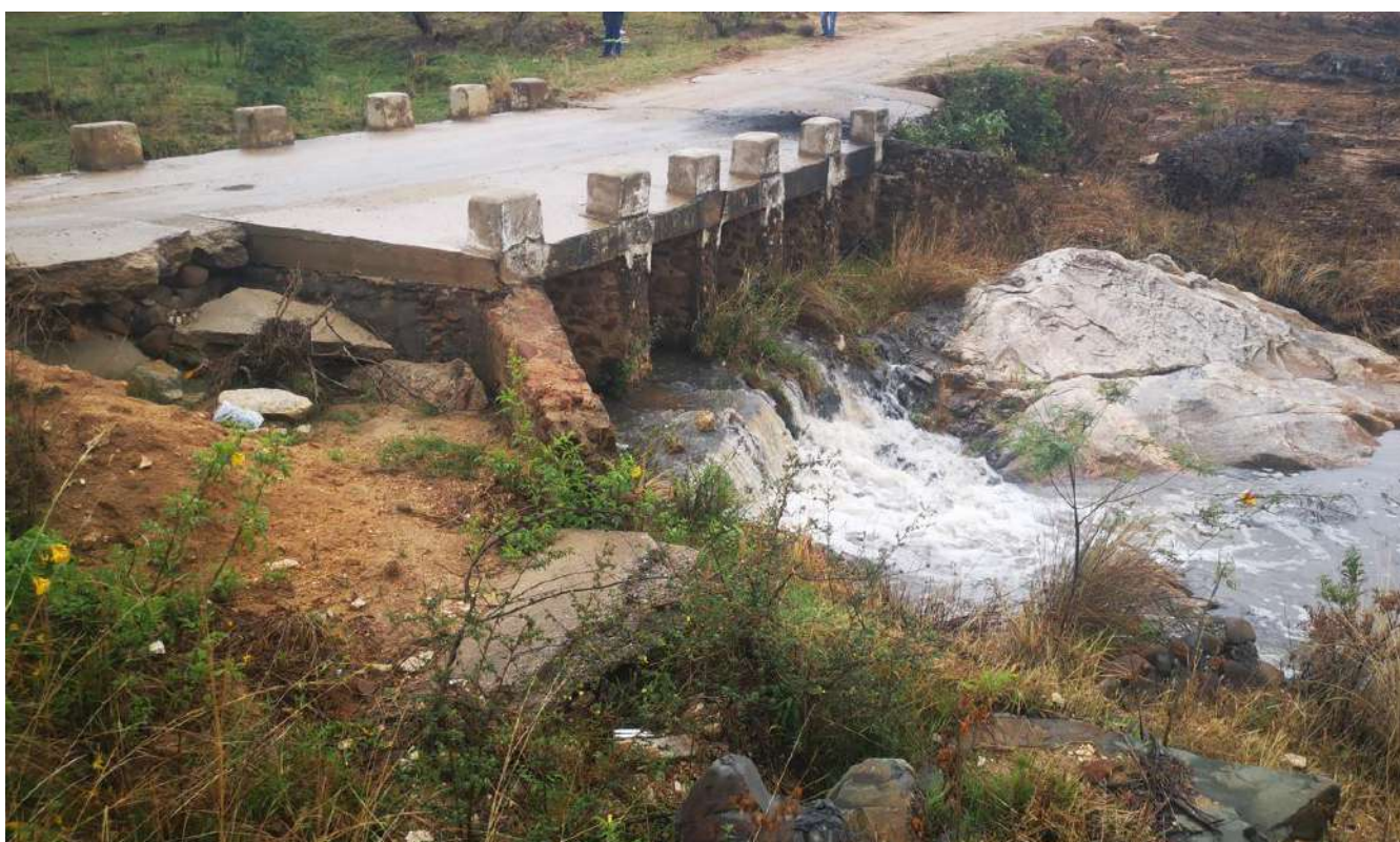
Figure 9 Stream 1 culvert 3 approach erosion
