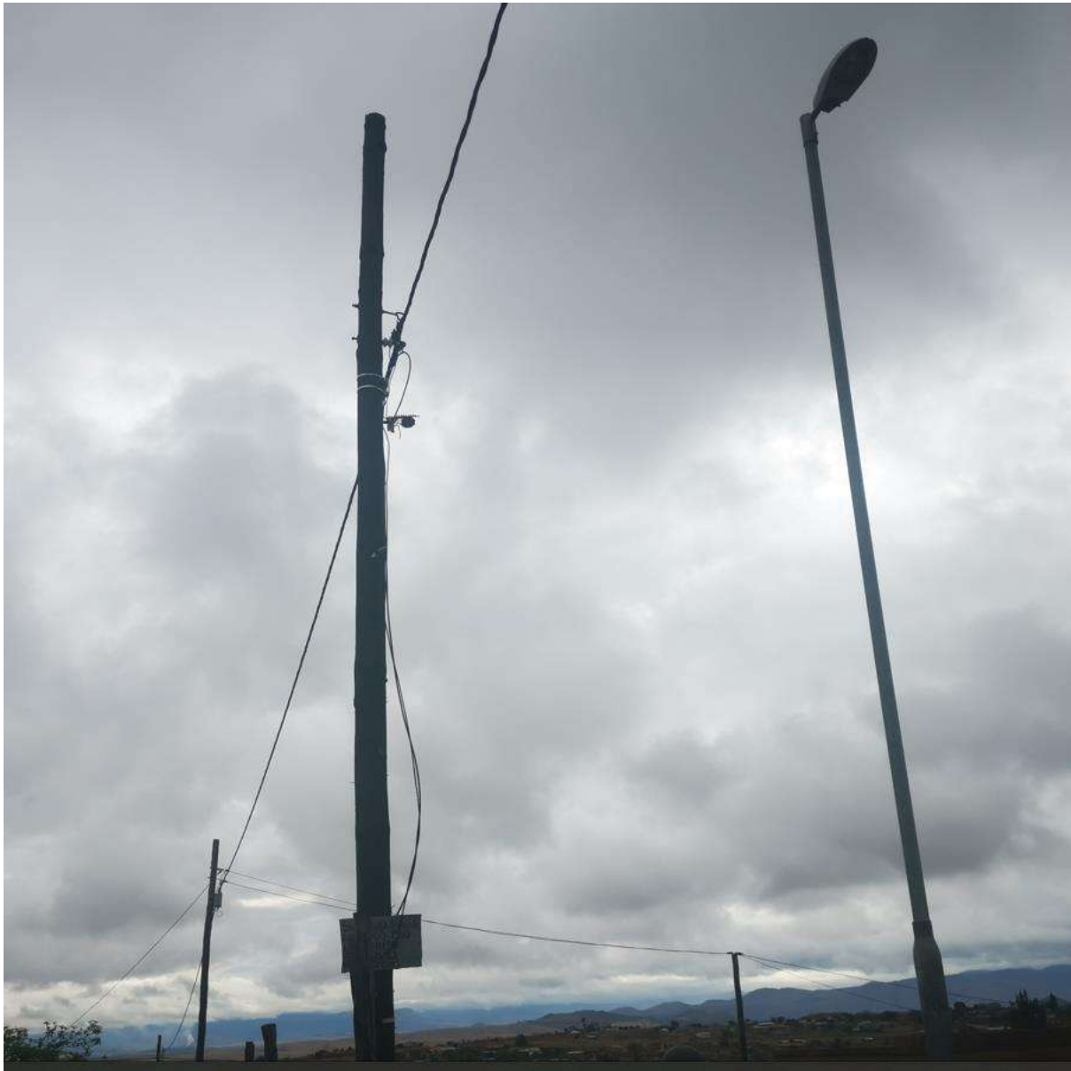
Figure 21 Electrical lines onsite
