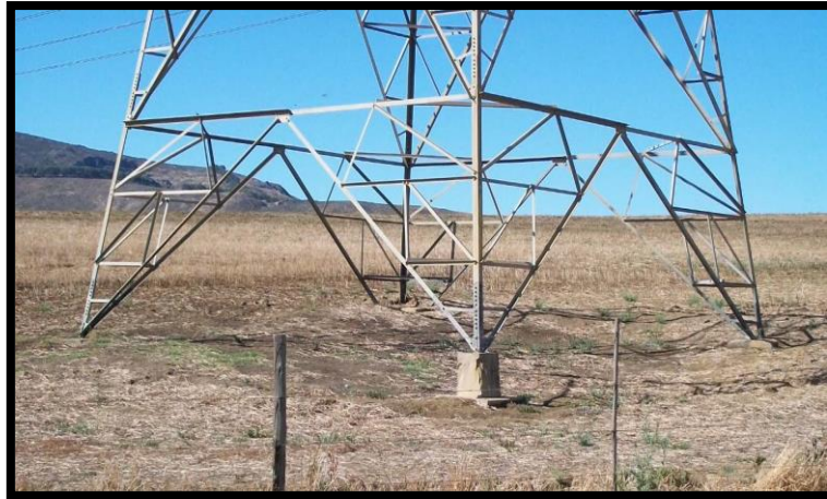
Photo 5.4: Typical dead man anchor foundations for guayed towers (Photo courtesy of Outeniqua Geotechnical Services, 2017).
