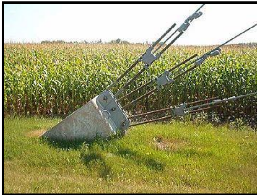
Photo 5.3: This Figure depicts the typical gravity foundation of lattice steel self-supported transmission towers (Photo courtesy of Outeniqua Geotechnical Services, 2017).
