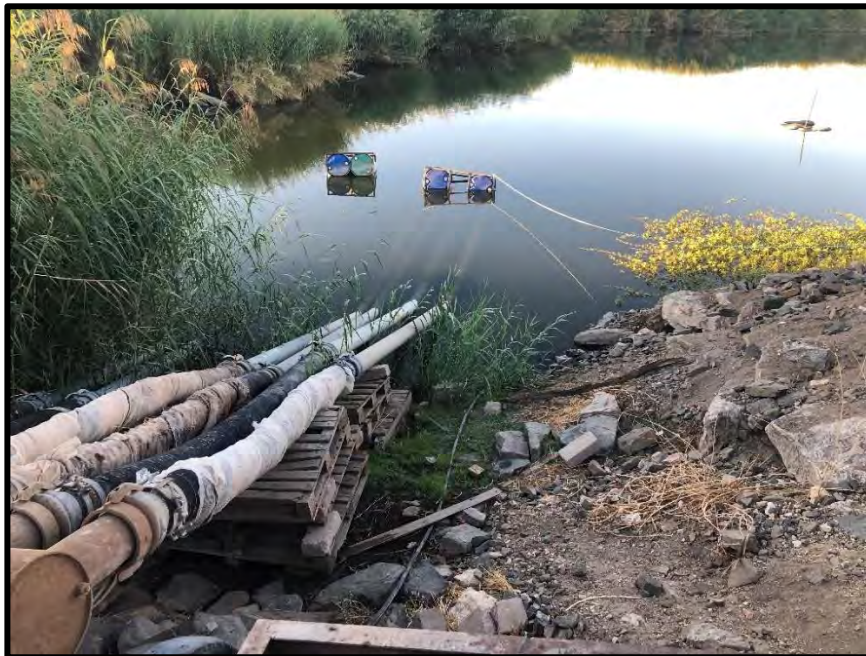
Figure 11: River pump station
