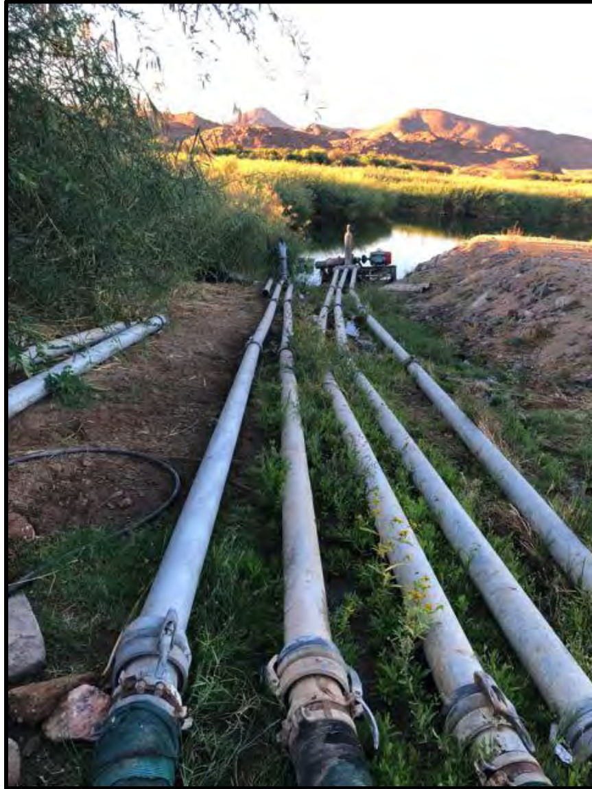
River pump station
