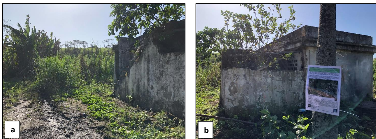
(a) View of the current pump dilapidated station; (b) Additional view of the current pump station.
