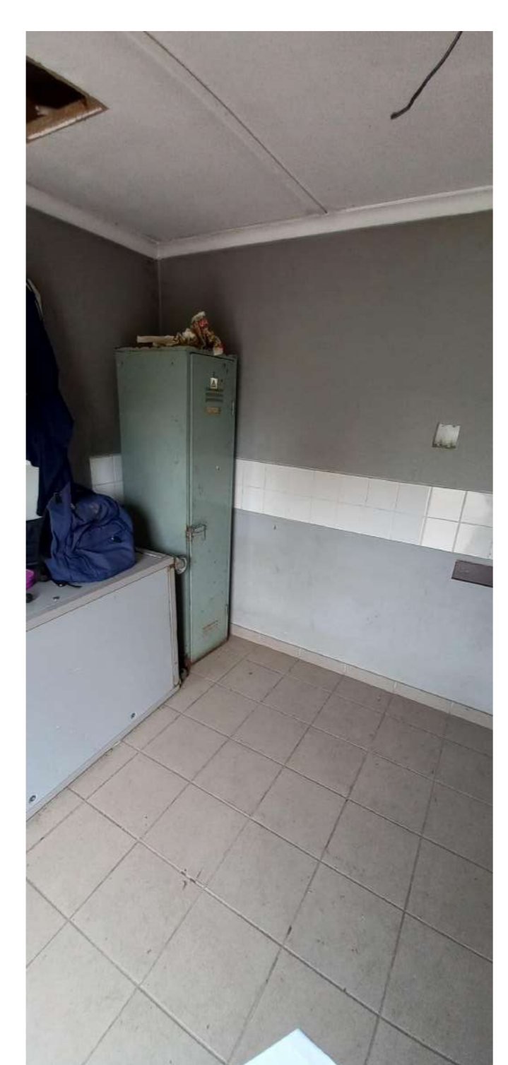
3. EXISTING SECURITY OFFICE (UNLAWFUL) - INTERNAL
