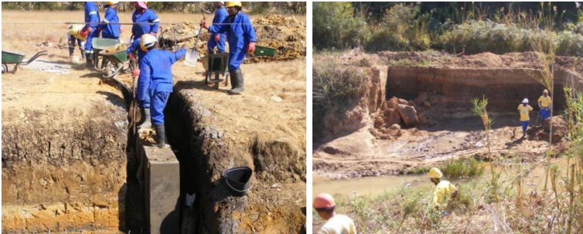
A buttress weir being built and a site being prepared by the Implementing agents
