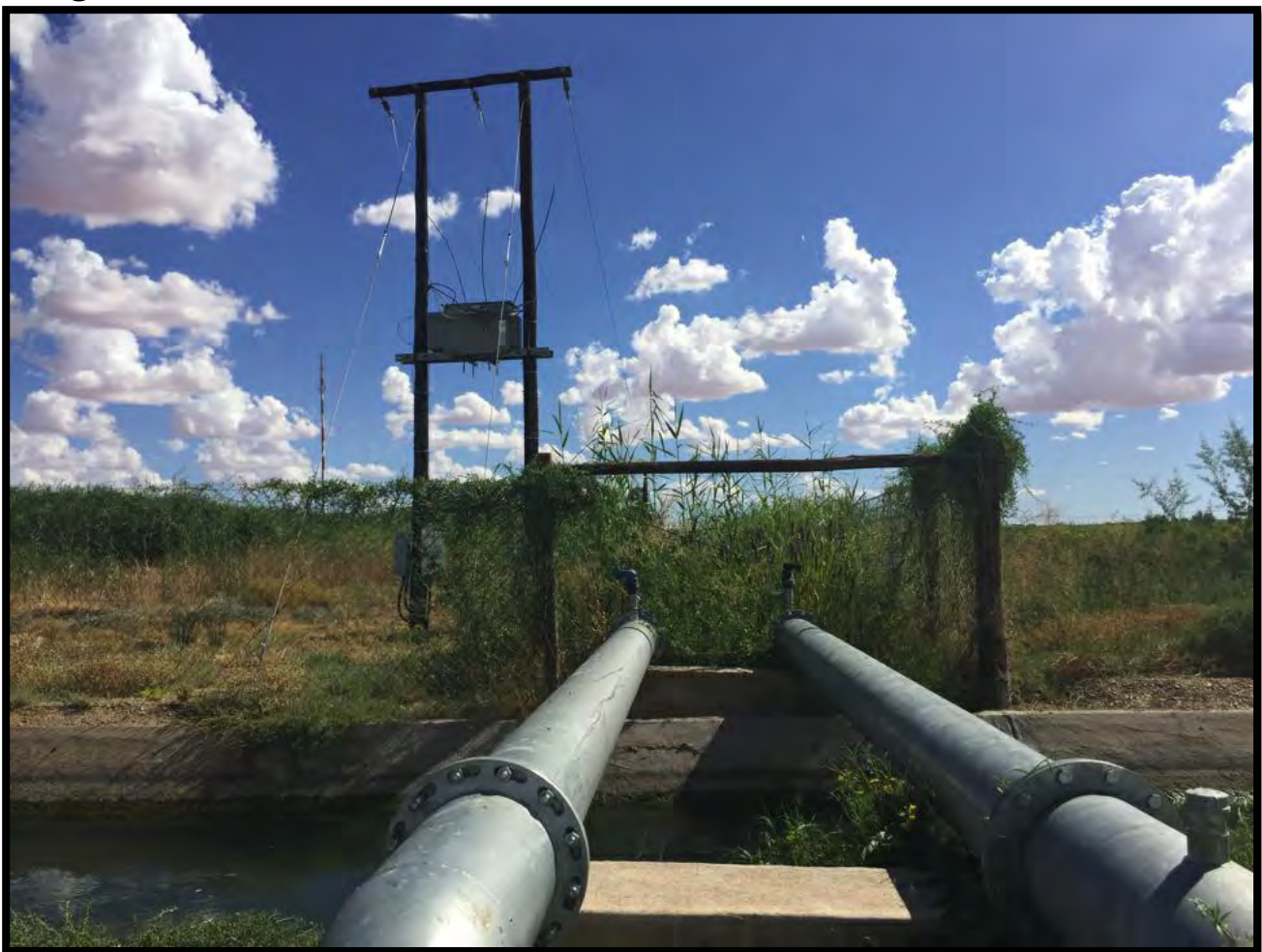
Figure 11: Electrical access point
