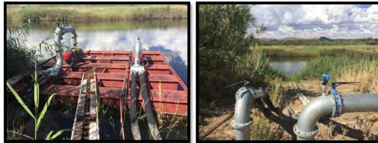
Figure 11: Photo's of pump station
