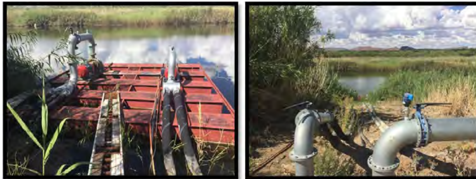
Figure 10: Photo's of pump station
