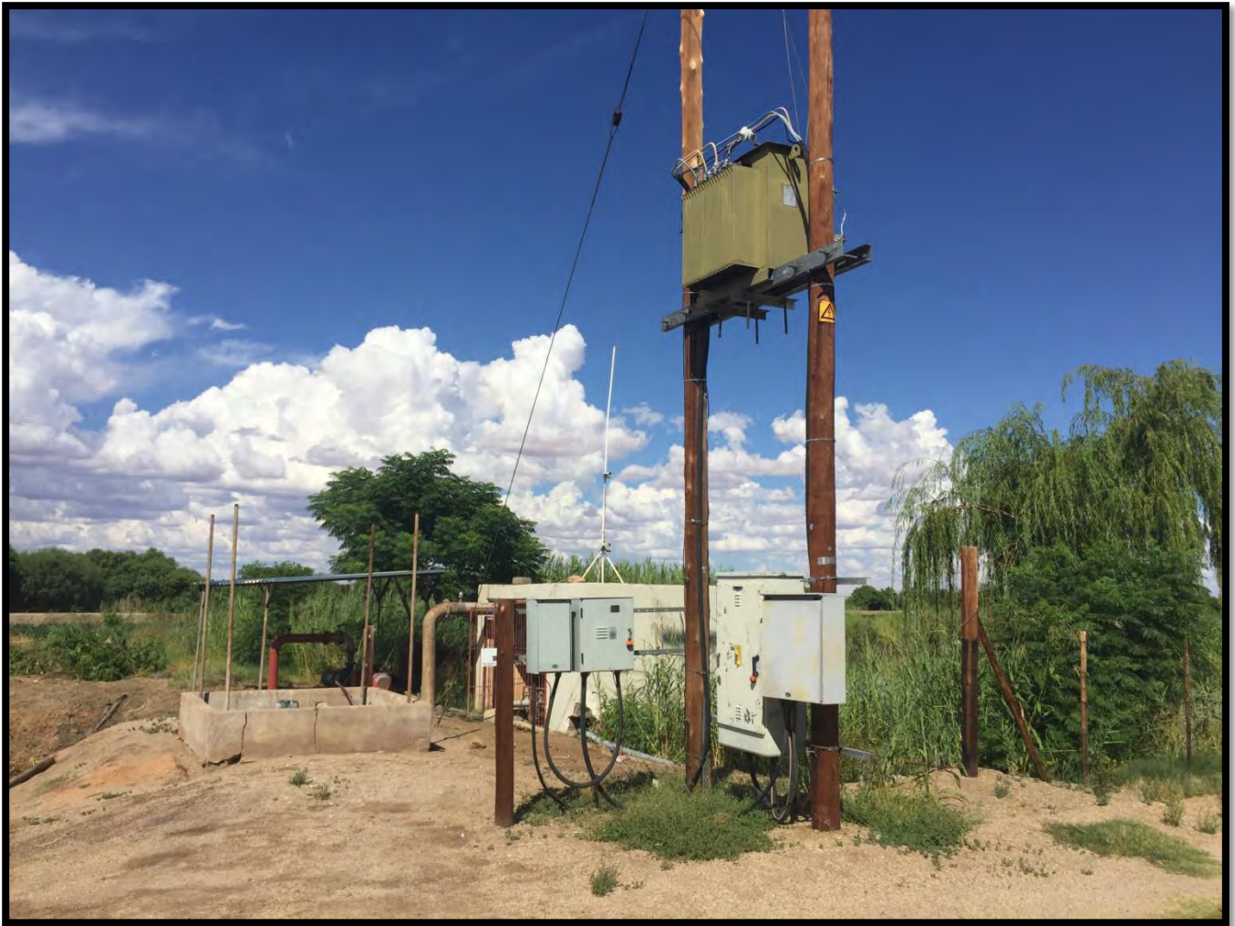
Electrical connection at dam
