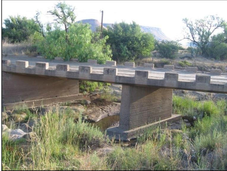
Figure 15. Existing bridge structure. Note the presence of wetland and riparian vegetation on the bed and banks
