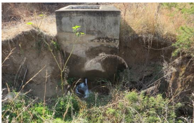
Existing stream crossing and impact due to leakage
