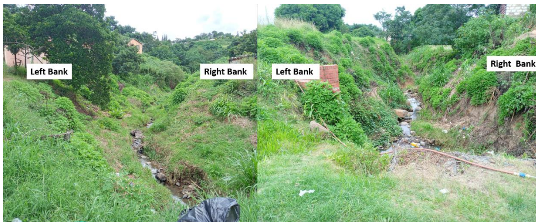
Photo 5-2: General Channel and Floodplain View of the Un-named Stream 2 at the Project Site
