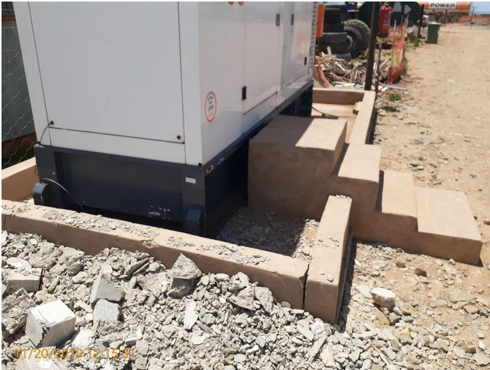
Photo Plate 7. Generator stored within bunded area.
