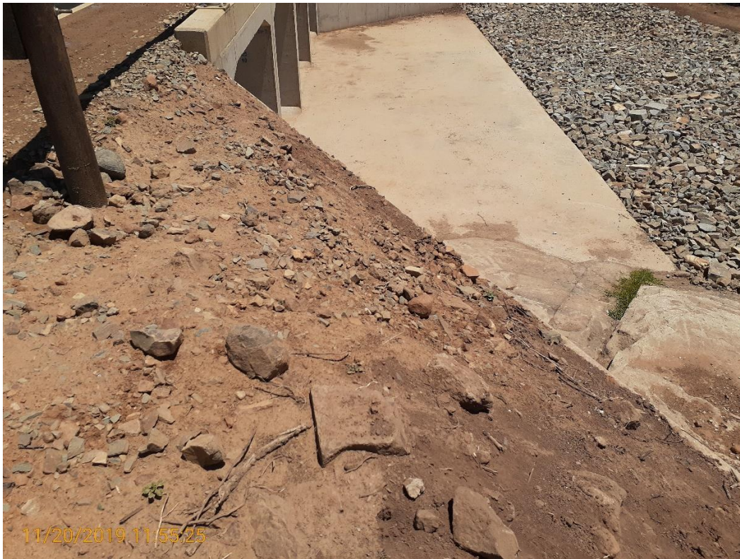
Photo Plate 1. Steep slopes next to the river crossing that would be prone to future erosion.
