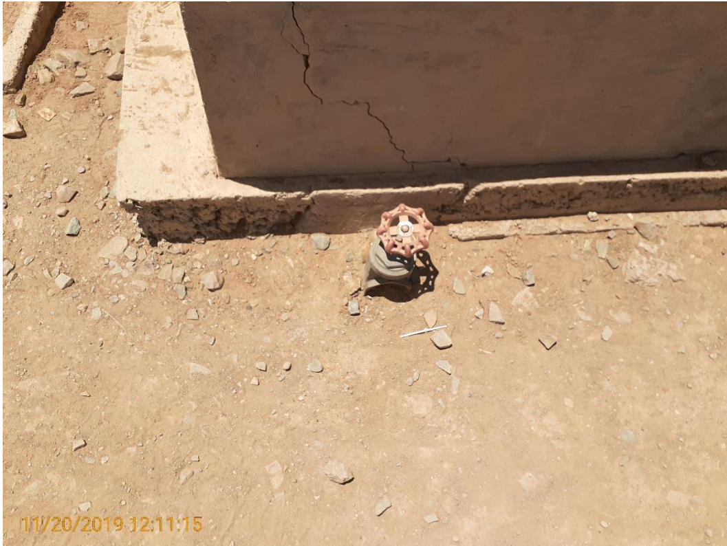
Photo Plate 3. Tap off system non functional at the bunded area. The pipe is full of ground.
