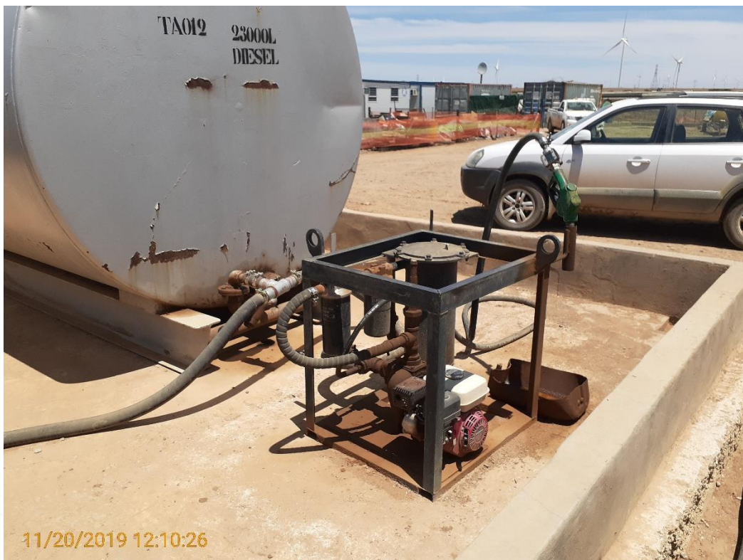
Photo Plate 2. Diesel tanks and pumps within the bunded area at the contractor's site camp.
