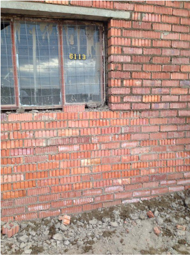
Images 004 & 005: Indicating damages to brickwork, roofing and gumpoles.
