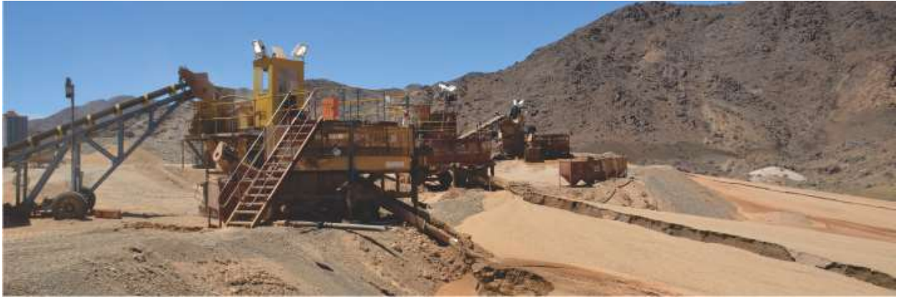
Photo 5: The current 3 x 16ft pans depositing fine tailings into the Oena Fine Tailings Dam
