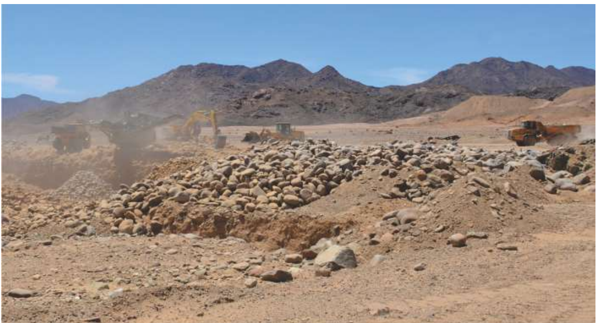
Photo 1: Current backfilling in the Oena East section. Backfilling has progressed extremely well with material obtained from reprocessing of existing main plant dump.
