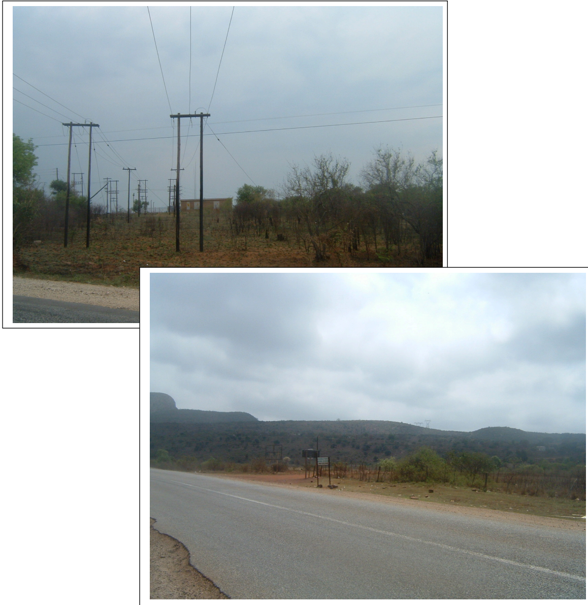
Figures 5 & 6- The Lemara Substation on Richmond 604KT from where the 132kV power line departs (above). The first stretch follows the northern shoulder of the R36 which runs between Ofcolaco and Hoedspruit (below).
