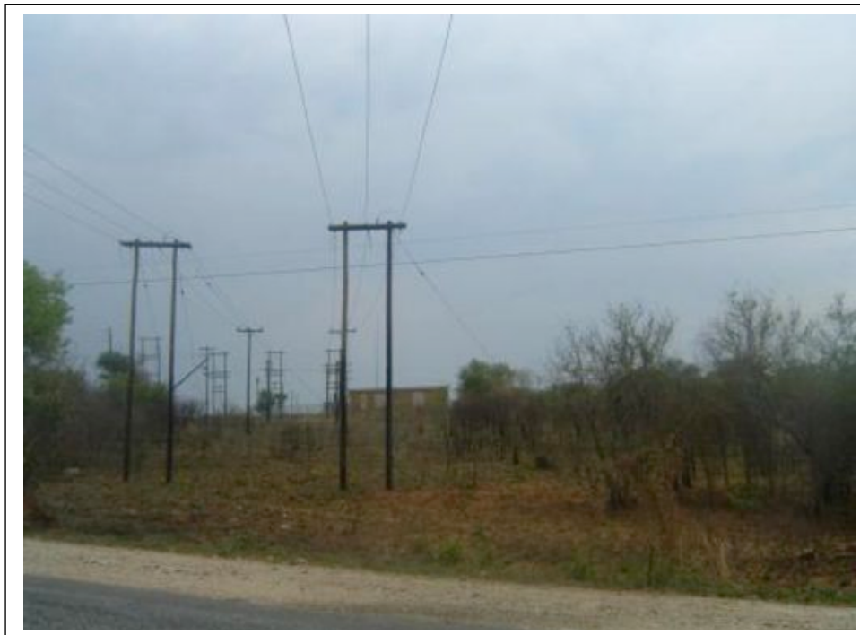
Figure 9- The Lemara Substation on Richmond 604KT where the proposed new 132kV Lemara-Leboeng power line commences (above).
