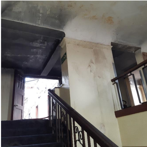
Picture 1 : RC roof over stairs. View from Staircase towards the entrance to the 2 nd floor
