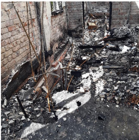
Picture 11 : Collapse of timber floor
