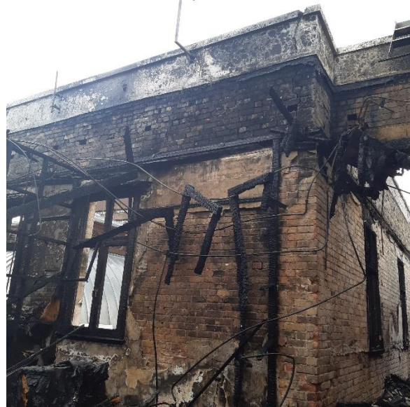
Picture 6 : Parapet wall – crack in wall
