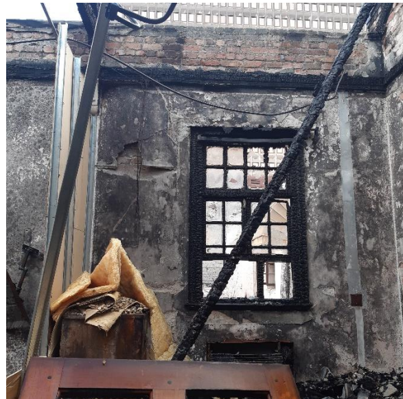
Picture 4 : View in one of the Offices – burned windows
