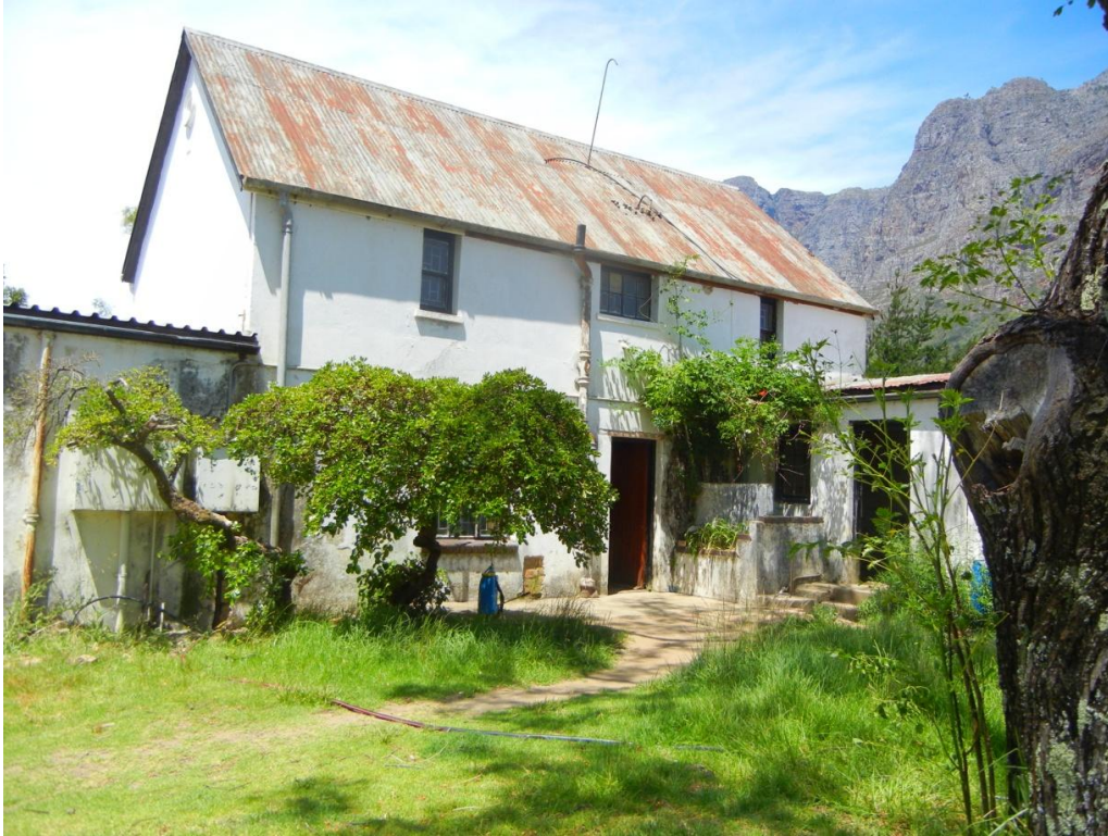
View of “Double storey Cottage’ in Kitchen Werf - Roof Sheeting to be replaced
