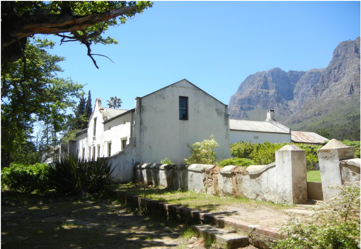
View of Old Bethlehem Homestead from Wine Cellar side – Roof sheeting to be replaced
