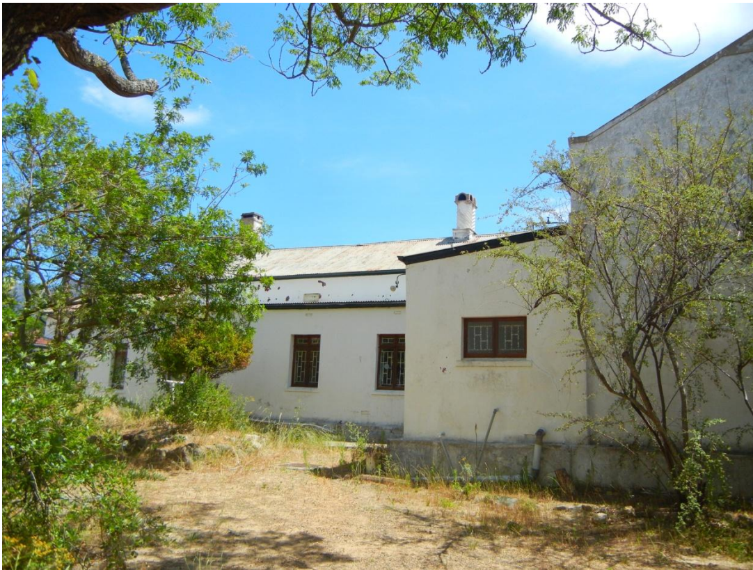
Kitchen Werf Side View of Homestead showing 19 th century Lean To additions
