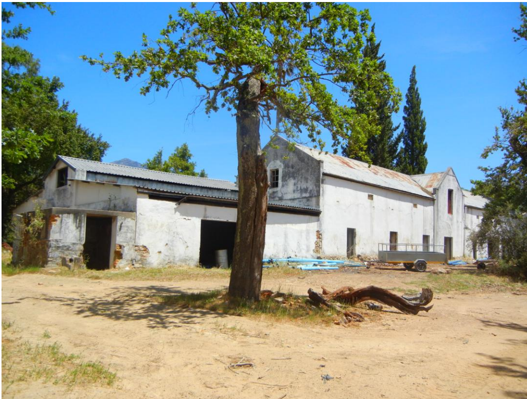
View of Large Shed (left) and Stable Building – Roof sheeting to be replaced on Stable building
