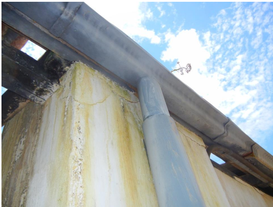
Miscellaneous Galvanized steel downpipes to be sorted out.
