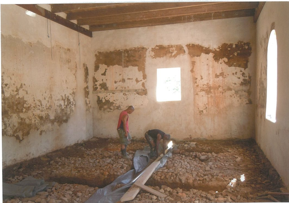
2. View towards Room C with a central trench (already filled) two trans-verse open trenches. The area of the blackened stones is marked "Hearth" (look W).
