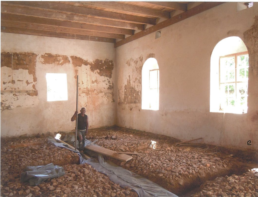
7. View towards Room C façade, with Trench e on the right (look W).
