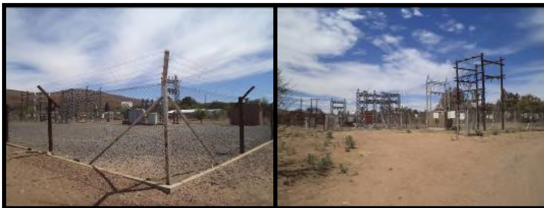
Figure 3: Existing Olifantshoek substation to be decommissioned
