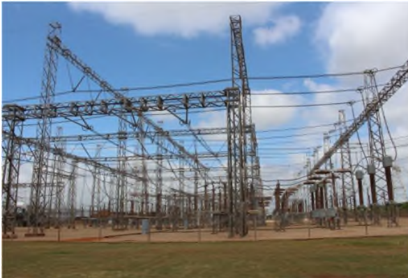
Plate 1 - Sub-station Bus Bars maximum height 10-15m
