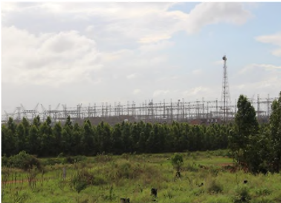
Plate 3 - Sub-station & Communication Tower
