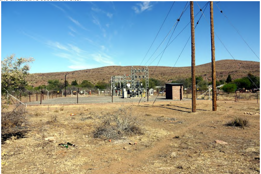
Plate 14 – VP4 looking west towards the existing substation.
