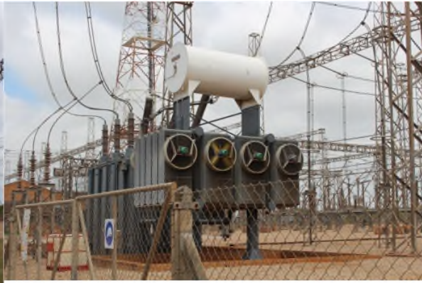
Plate 2 – Transformer with oil storage tank above.
