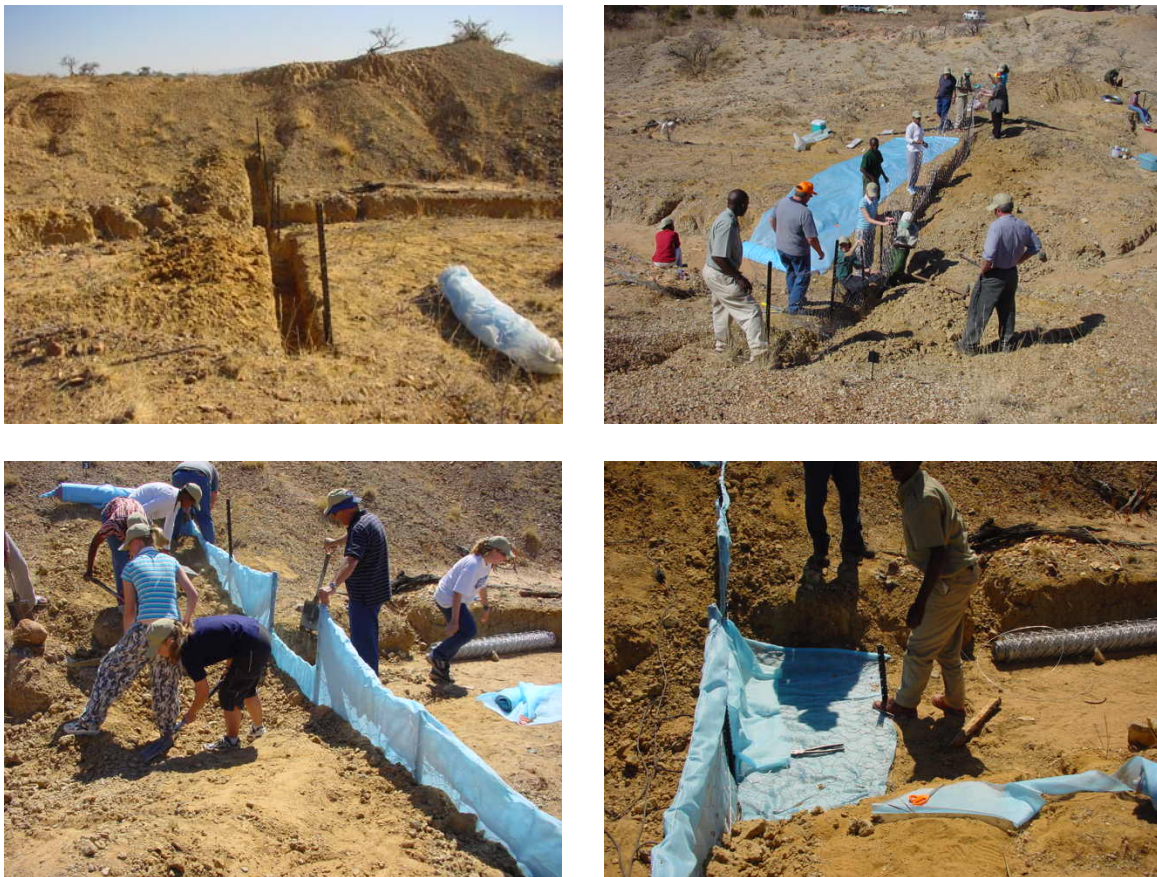
Figure 6: The photographs show the steps in the construction of a silt-screen. Girls from two schools in Pretoria on the Mabula Game farm carried out this exercise. In photo 1 the trench is dug across the erosion channel and Y standards are placed to form the main part of the structure. In photo 2 the Y standards are connected with stay wires and covered with wire mesh. The structure is then covered with a biodegradable geo-textile in photo 3. In photo 4 the structure is completed by adding an apron, made of geo-textile and wire mesh.
