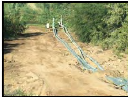
Figure 10: Photo's of pump station
