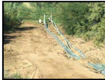
Figure 11: Photo's of pump station
