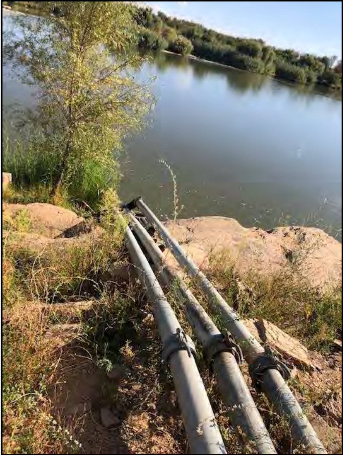
River pump station
