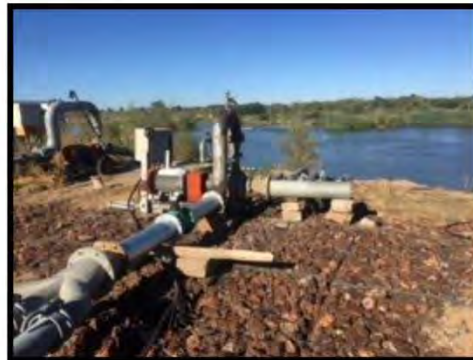
Figure 14: Photo's of pump station
