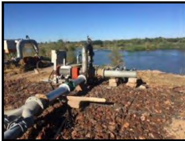
Figure 10: Photo's of pump station
