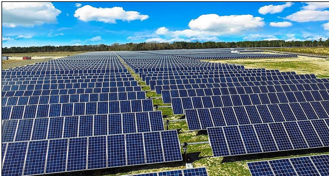
Figure 2.1: Typical example of solar PV array
