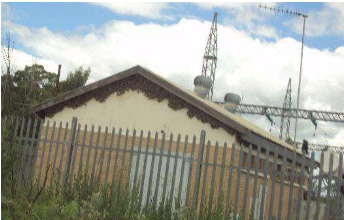
Figure 19: View of northern end of the substation building, showing swallow/ swift colony nests
