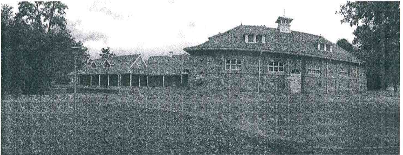
Front elevation of Ward 6- OT building and OT hall after roof renovations
