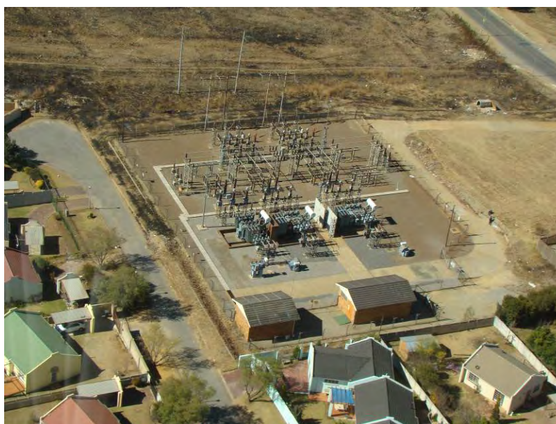
Figure 3.11: Example of a typical 132kV substation
