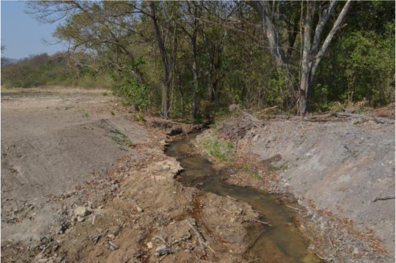
FIGURE 29: A WETLAND IMPACTED BY RECENT ROAD CONSTRUCTION ACTIVITIES ALONG THE PORTION OF THE EXISTING SERVITUDE THAT WOULD LINK THE P166 WITH THE R40 TO THE NORTH OF THE RIVERSIDE MALL AND N4 BYPASS IN MBOMBELA
