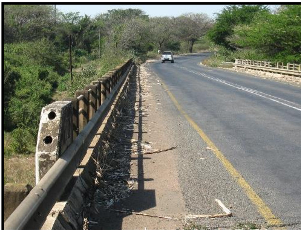
Figure 8. Road bridges on the area earmarked for rehabilitation on the P230 are all younger than 60 years old.
