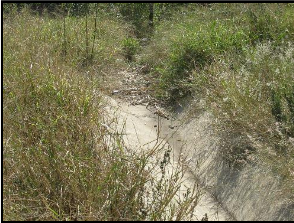
Figure 9. The existing culvert of the P230 is younger than 60 years old.
