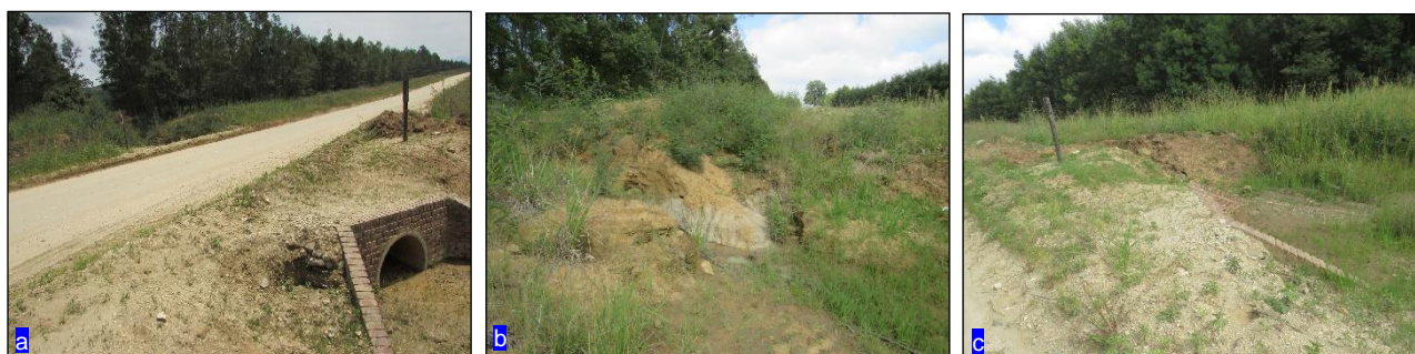
Figure 10: (a): Image showing existing structure at RC1 and P303 road. Note sedimentation of pipe; (b): Image showing upstream characteristics of the existing P303 structure (c): Additional image showing downstream of RC1.
