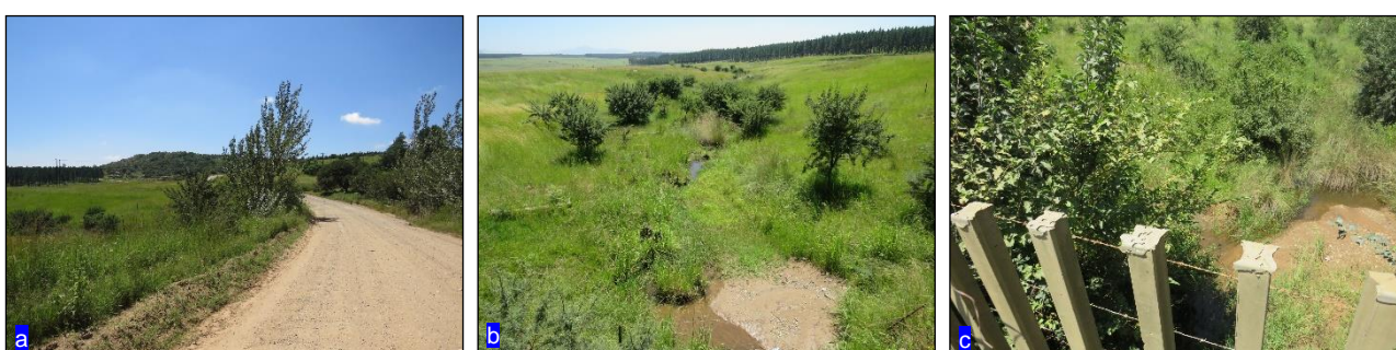
Figure 12: (a): Image showing P303 approaching RC3. (b): Photograph showing downstream characteristics at RC3 (c): Image showing upstream characteristics at RC3 and associated deteriorated infrastructure to be repaired. Note, this existing structure, at RC3, will only be repaired and not upgraded .
