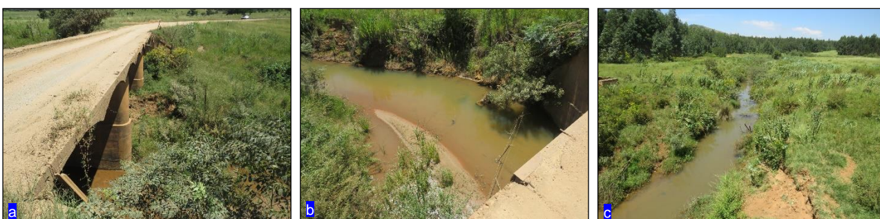
Figure 13: (a): Image showing existing infrastructure at RC4 (b): Image showing downstream characteristics at RC4 (c): Image showing upstream characteristics at RC4.
