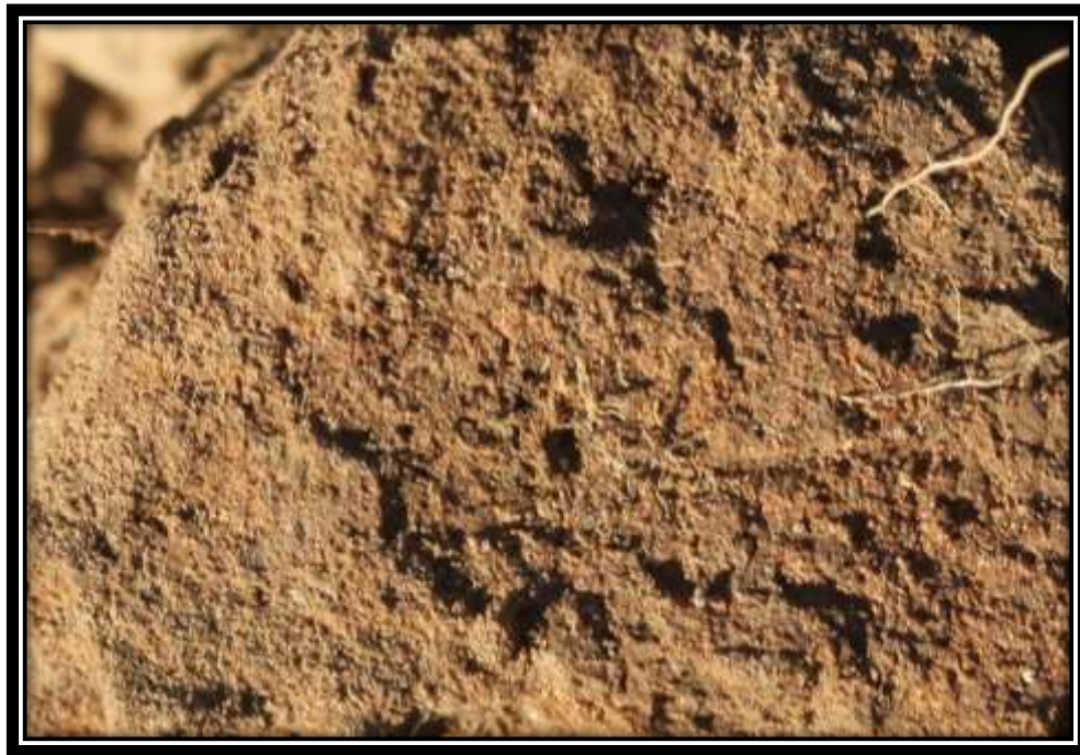
Photograph 17: Soil sample at a furrow at the site. The furrows at the site appear to be dysfunctional at present.
