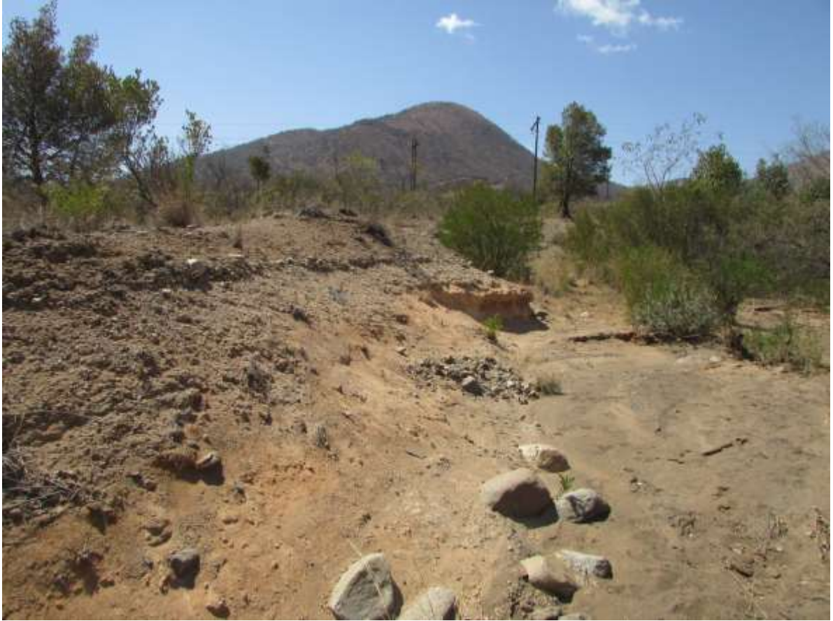
Figure 15: A view of a section of the erosion donga near OC3.
