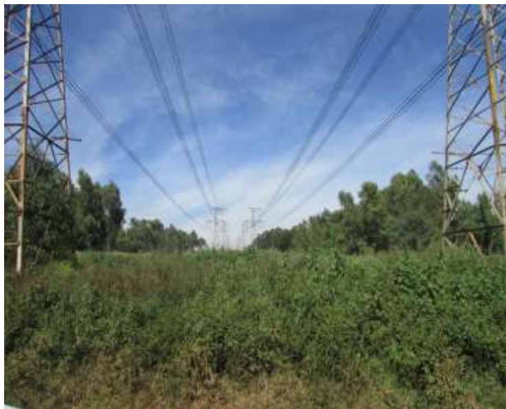
Fig.4: Another view showing the ESKOM Powerline & Pylons over a section.
