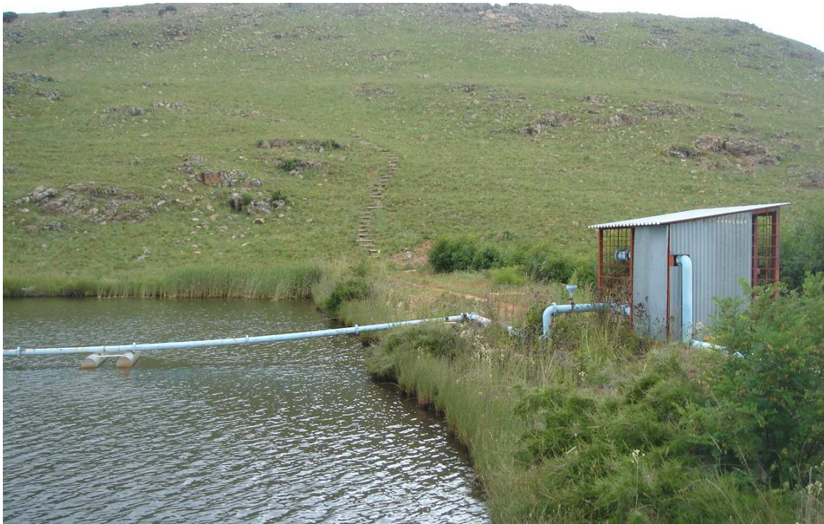
Existing pump station with Suikerboskop in the background
