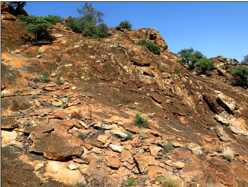
Figure 15. Scabby weathered surface of Clarens sandstone with spalling of platy blocks and flakes, Site 1 study area.
