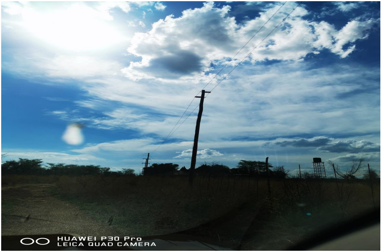
Figure 8: Existing powerline in the project area
