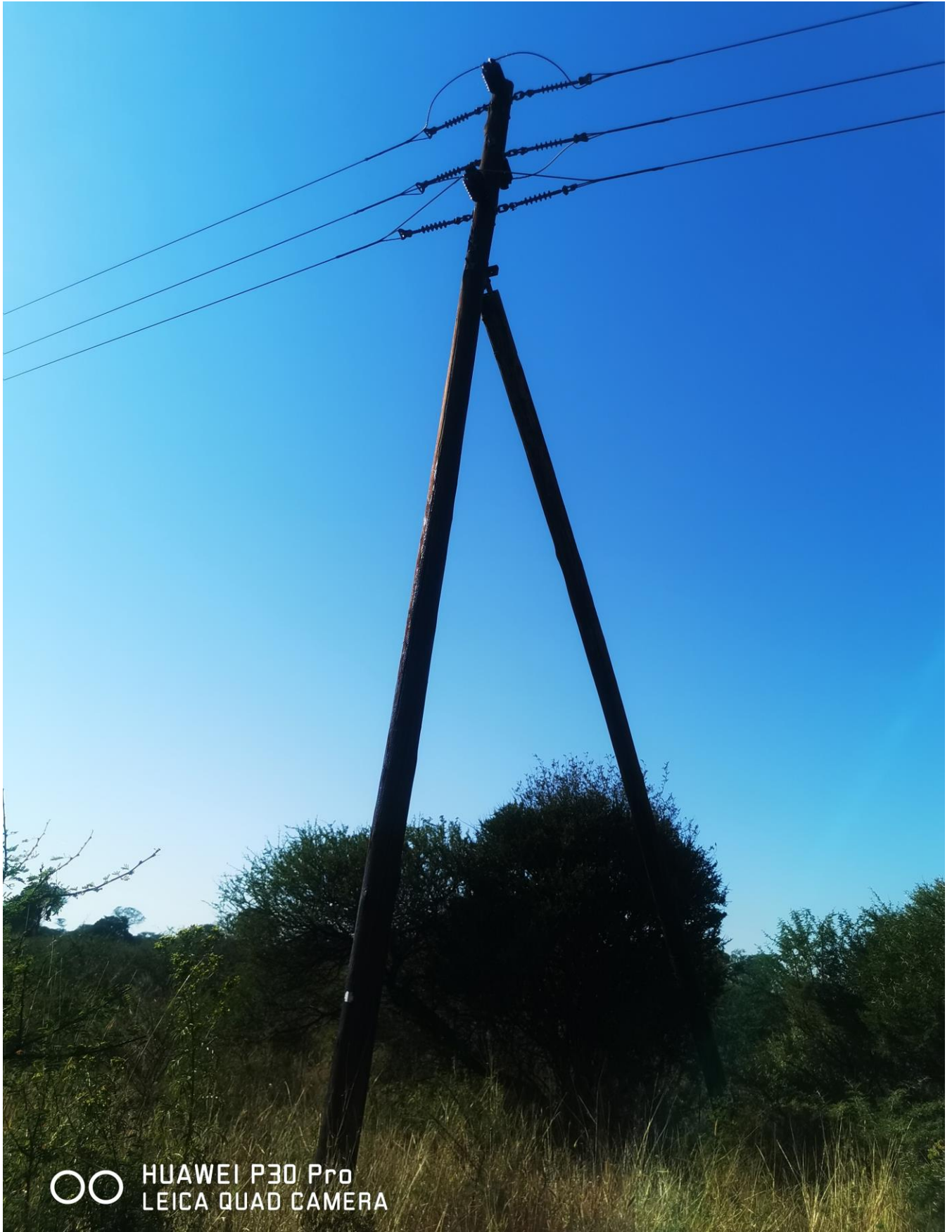
Figure 2: Existing Electrical Infrastructure in the project area
