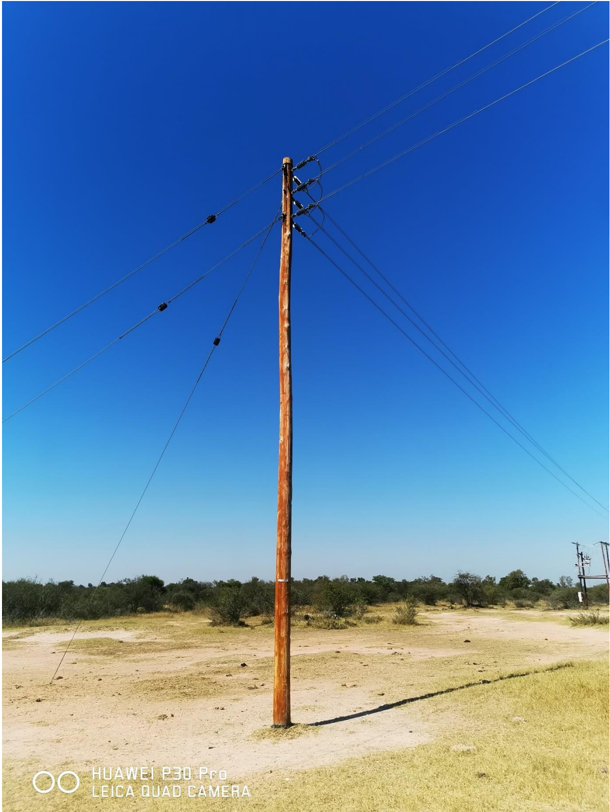
Figure 2: Existing Electrical Infrastructure in the project area
