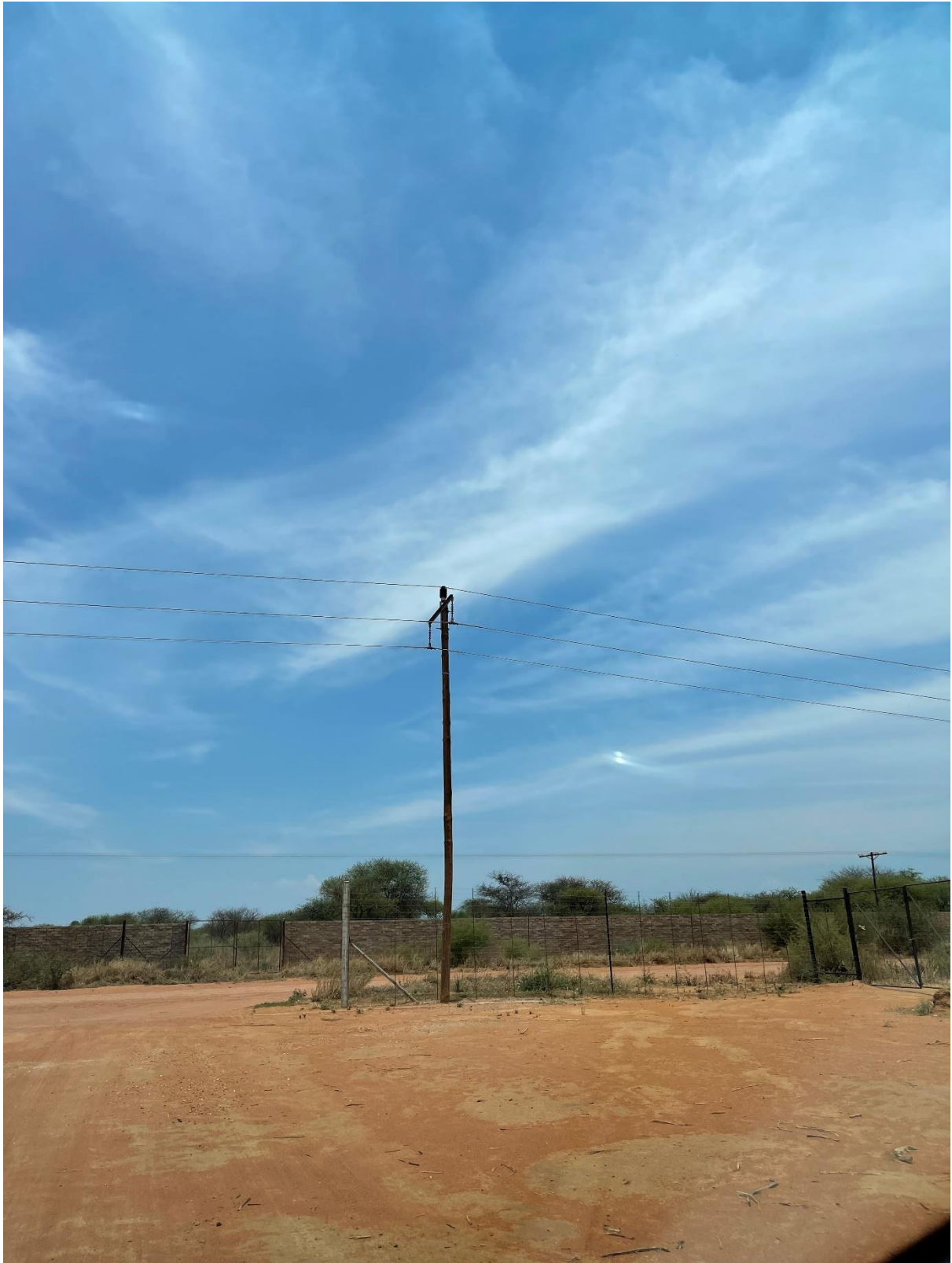
Figure 2: Existing Electrical Infrastructure in the project area
