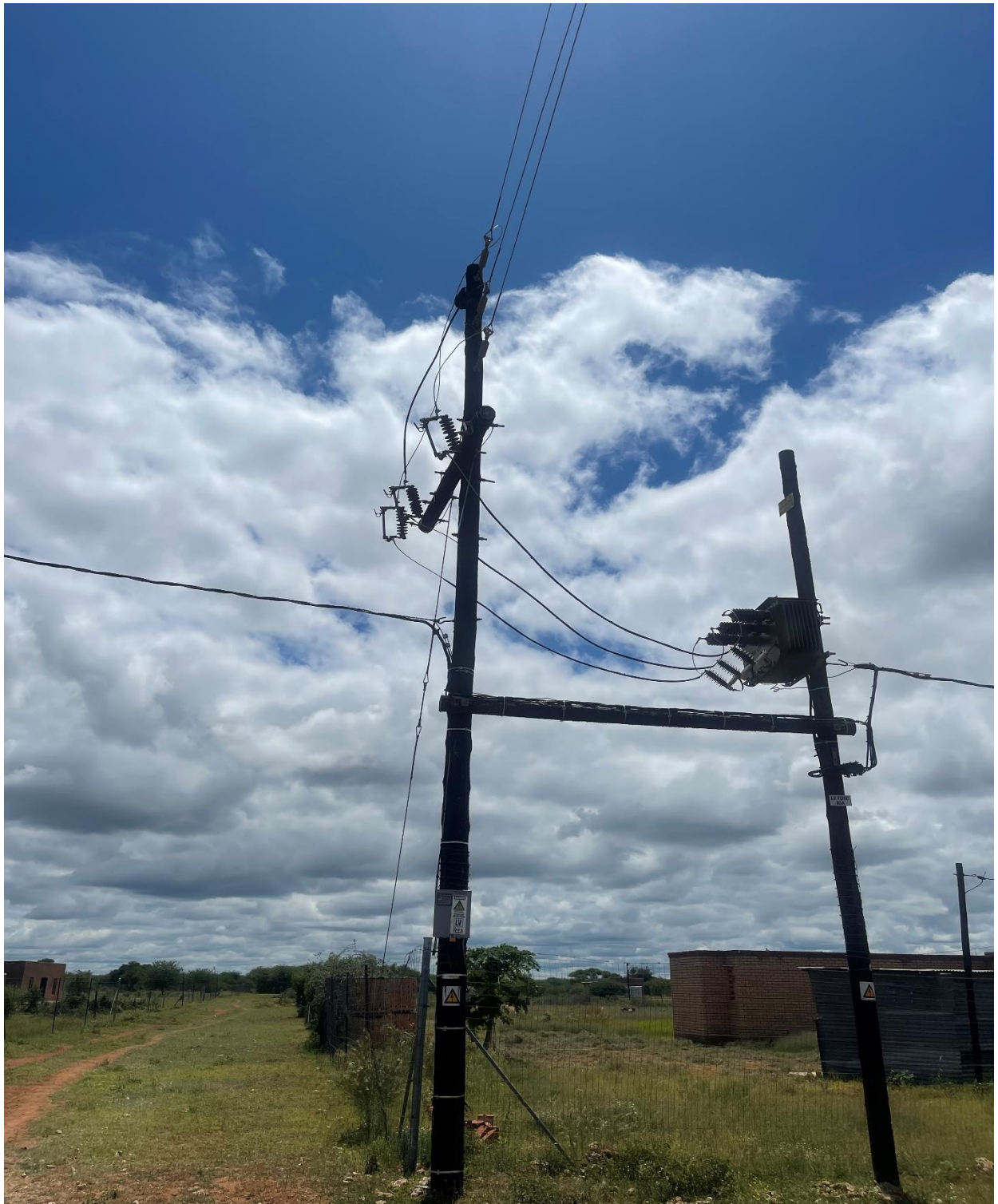
Figure 1: Picture showing existing electricity in the study area
