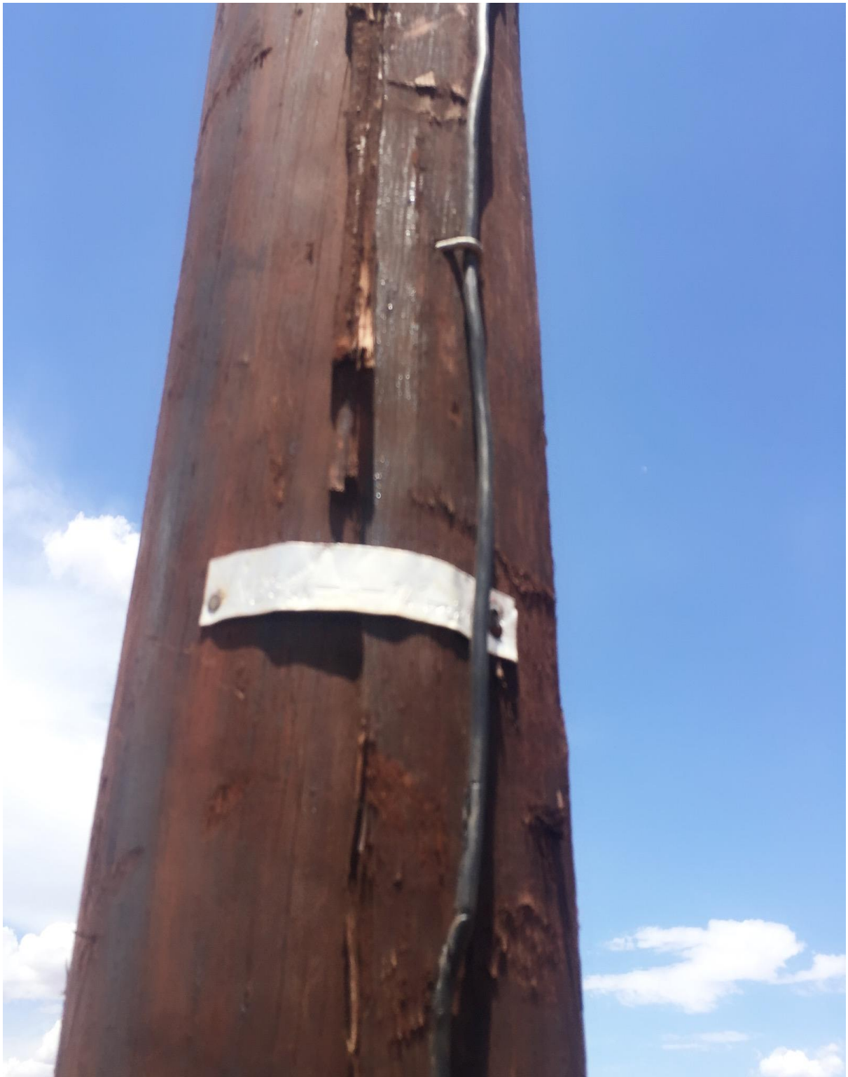
Figure 7: Picture showing existing electricity in the project area
